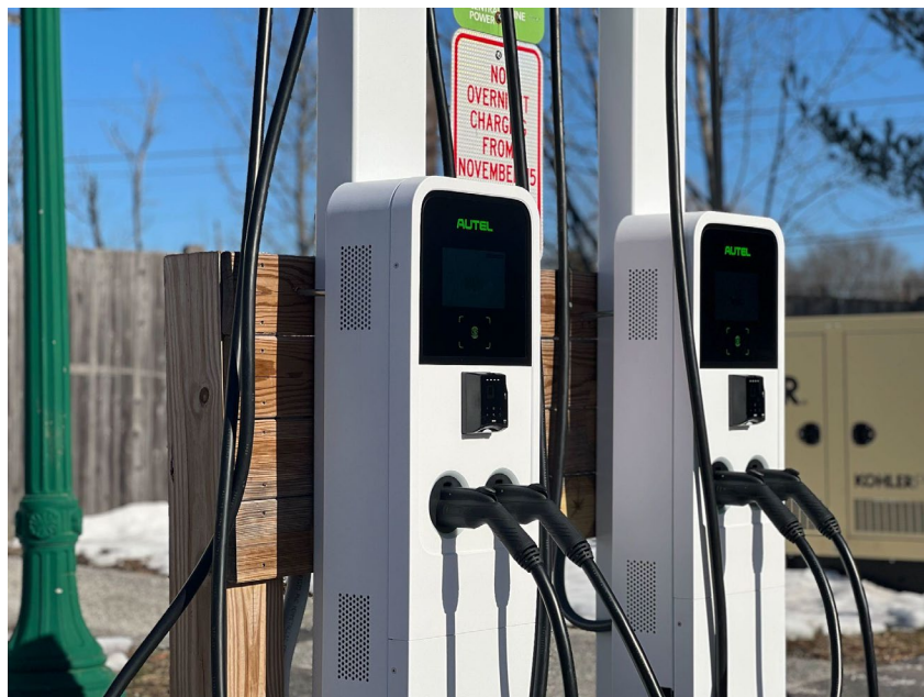
Public EV Chargers at Town Hall. Source: Town of Yarmouth
